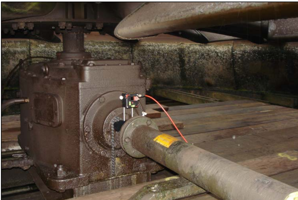
The beam hits the detector that is mounted on the gearbox for shaft to shaft alignment.
