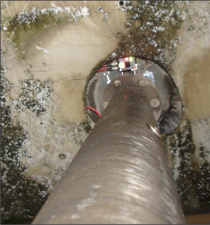
The laser beam from the motor shaft passes through the opening in the cooling tower wall.
